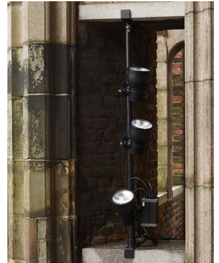
Dom Tower, Utrecht, Lighting fixed in tension
